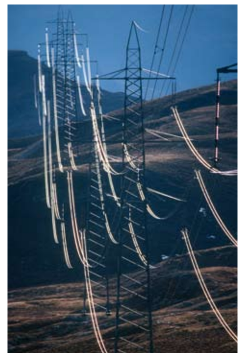
220 kV overhead transmission line near Laax (canton of Grisons).
