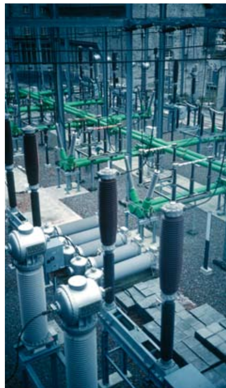
In addition to high-voltage power lines, sub-stations, too, produce relatively intensive magnetic fields within their fenced-in area.
